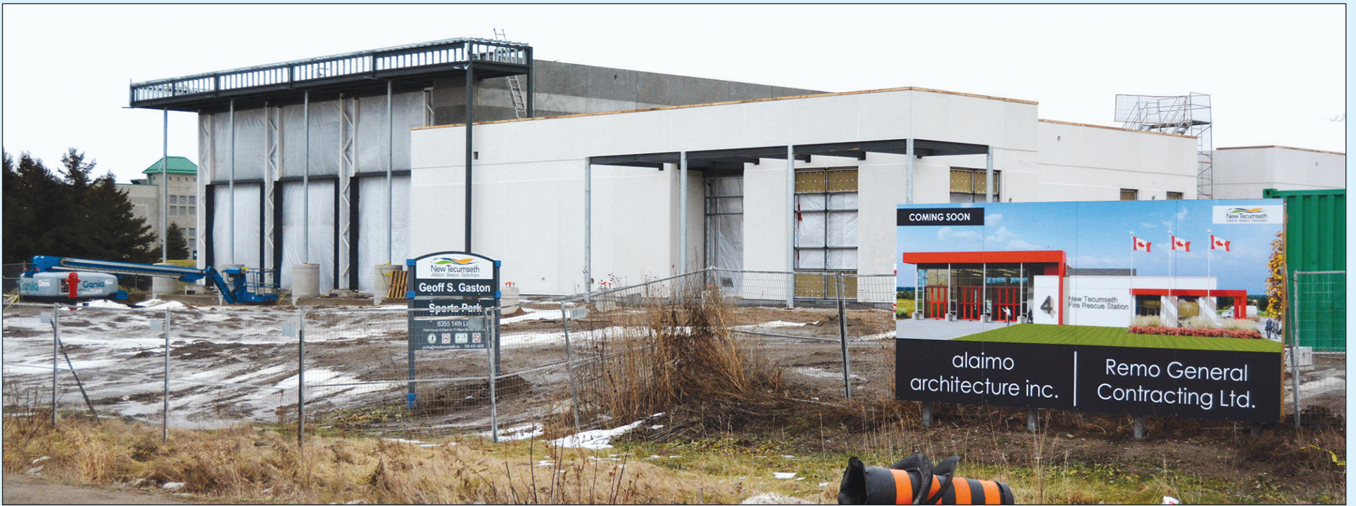
WORK CONTINUES – Work on the new New Tecumseth Fire Station 4 continues to move forward. The 12,600 sq. ft. facility will meet the need for expanded fire and rescue service as the Town grows. The new fire station is expected to open in fall 2026. BRIAN LOCKHART PHOTO
